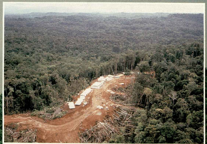
Fuel and plant equipment for the project is barged over 1200 km to Kiunga from Port Moresby; inset anti-clockwise from above: road construction from Tabubil to Mt Fubilan; road gangs sleep on the job in temporary camps; the road was cut through 135 km of virgin bush; traditionally the way to cross the raging streams in the mine area
