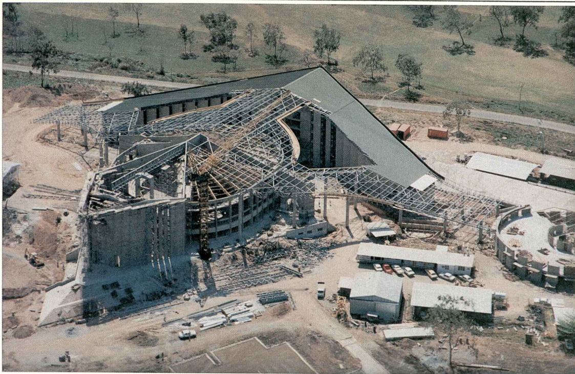
Parliament House - Port Moresby Roof Steelwork fabricated and erected by Hornibrook Constructions Pty Ltd. Protection Treatment: Abrasive Blast clean to Australian Standard 1627.4 Class 2.5 followed by Dimetcote 5 Inorganic Zinc Silicate to 75 micron dry film thickness.
