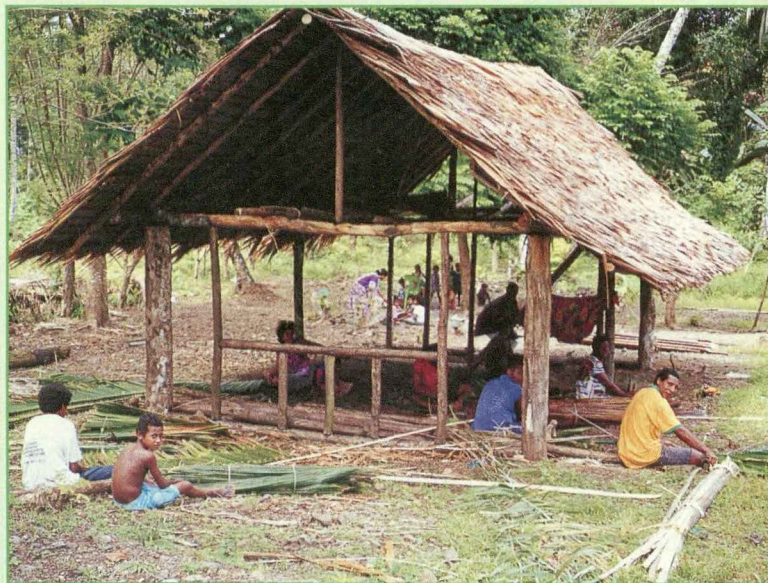
Below: An elementary classroom being built with bush materials by the community
