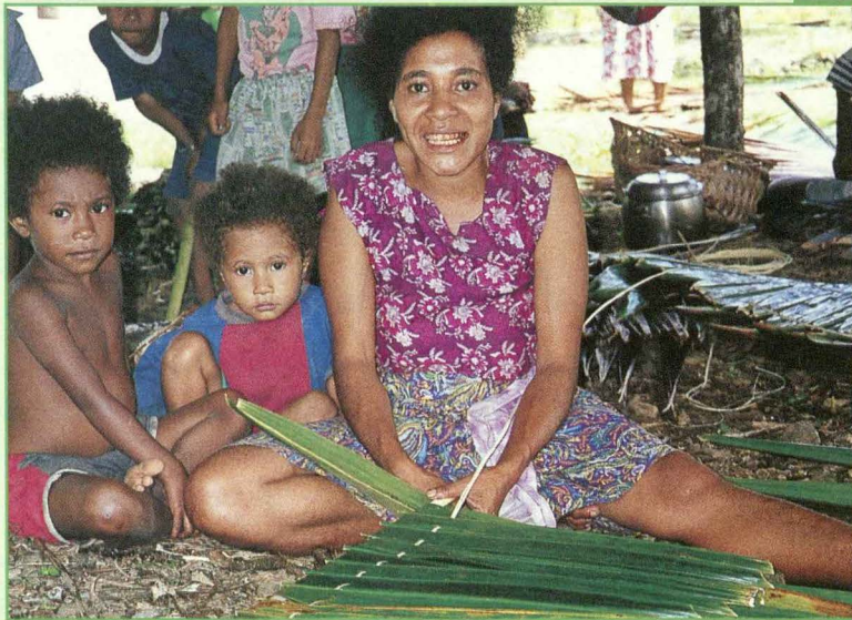
Above: A parent helps construct roofing for a new classroom at Gopaya Elementary School. Her two young children look on.
