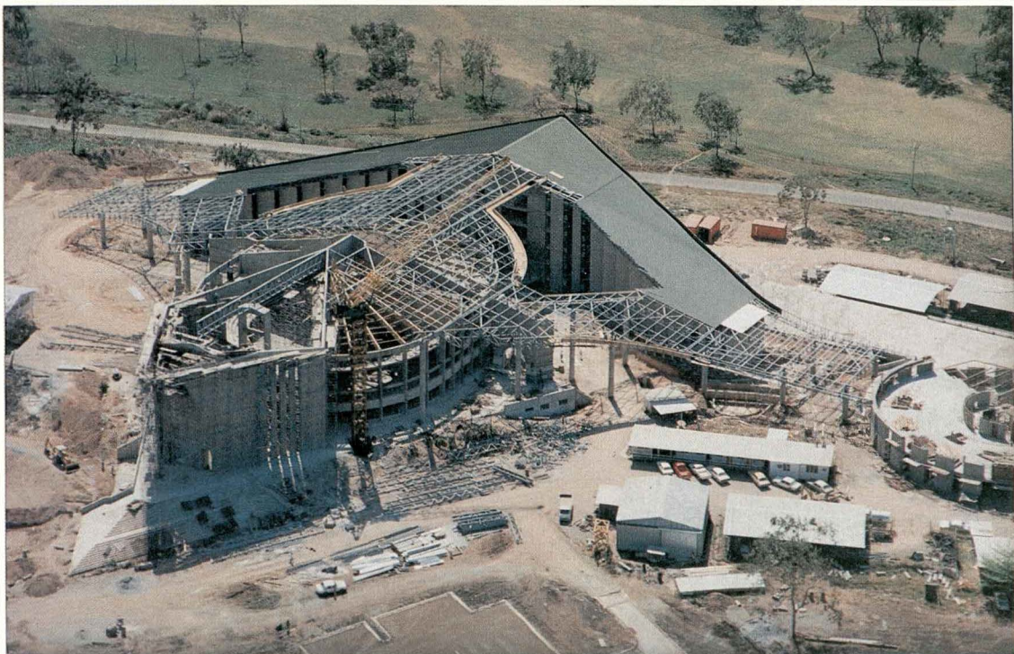
Parliament House - Port Moresby Roof Steelwork fabricated and erected by Hornbrook Constructions Pty Ltd. Protection Treatment: Abrasive Blast clean to Australian Standard 1627.4 Class 2.5 followed by Dimetecote 5 Inorganic Zinc Silicate to 75 micron dry film thickness.
