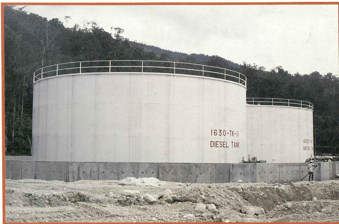
Two tanks - part of a large installation of bulk storage at Kiunga and Tabubil, Papua New Guinea for OTML. Tanks contain water and diesel fuel. Protective treatment of internal and external surfaces included Zincolite 120 - inorganic zinc silicate primer, top coated with Armourcote 418 and Amercoat 383HS - high solid epoxys.
