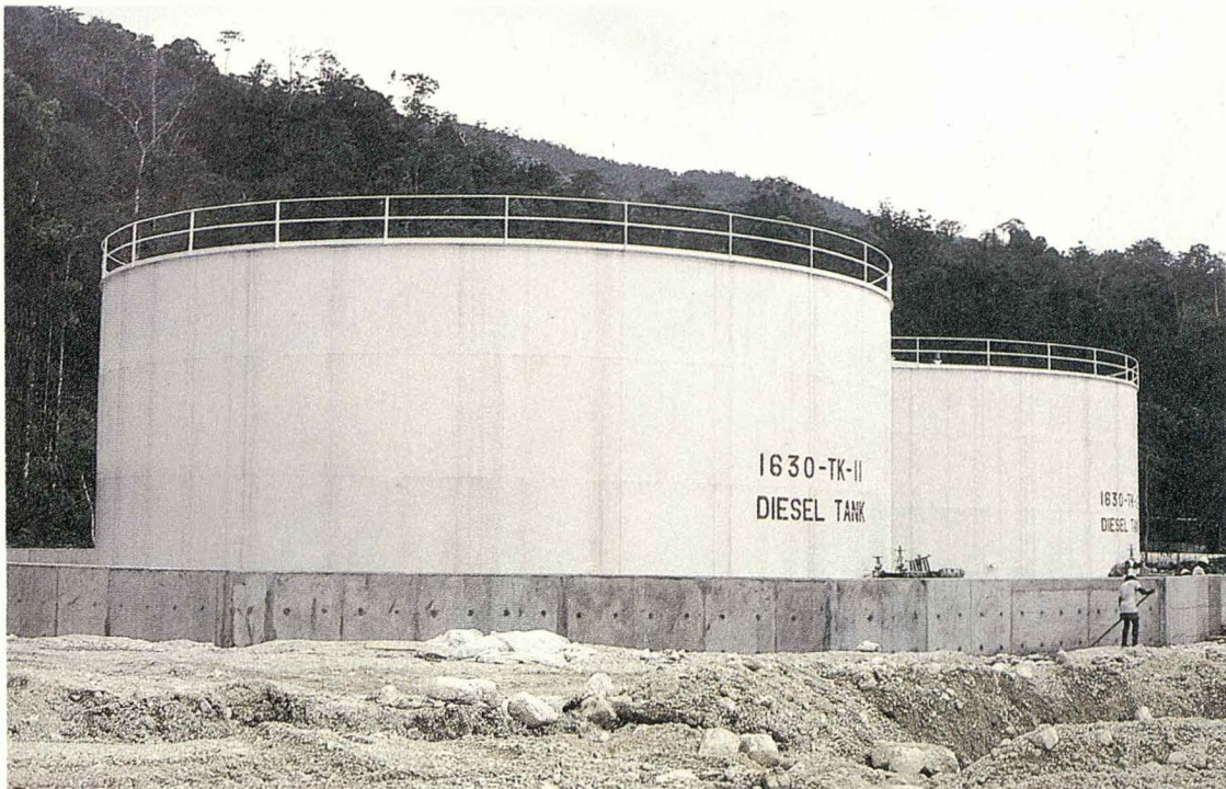
Two tanks — part of a large installation of bulk storage at Kiunga and Tabubil, Papua New Guinea for OTML. Tanks contain water and diesel fuel. Protective treatment of internal and external surfaces included Zincilate 120 — inorganic zinc silicate primer, top coated with Armourcote 418 and Amercoat 383HS — high solid epoxys.
