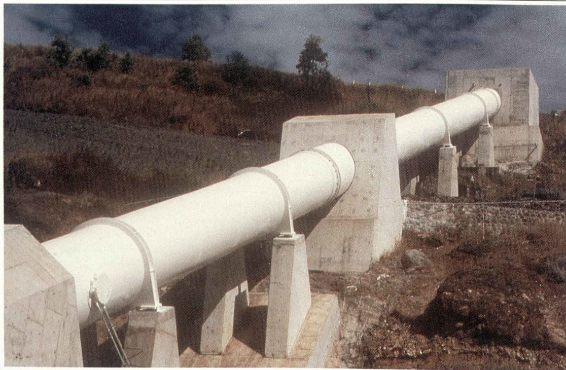
A section of Rouna 4 Penstock, near Port Moresby. 2.2 metres diameter, 300 metres long. Internal surfaces treated with 400 micron film thickness of Tarsel, Standard tar epoxy. External surfaces 75 micron film thickness of Dimetcote 5, inorganic zinc silicate and 75 micron of Unilite 400, poly vinyl chloride. Application by: Hornibrook Constructions Pty Ltd.
