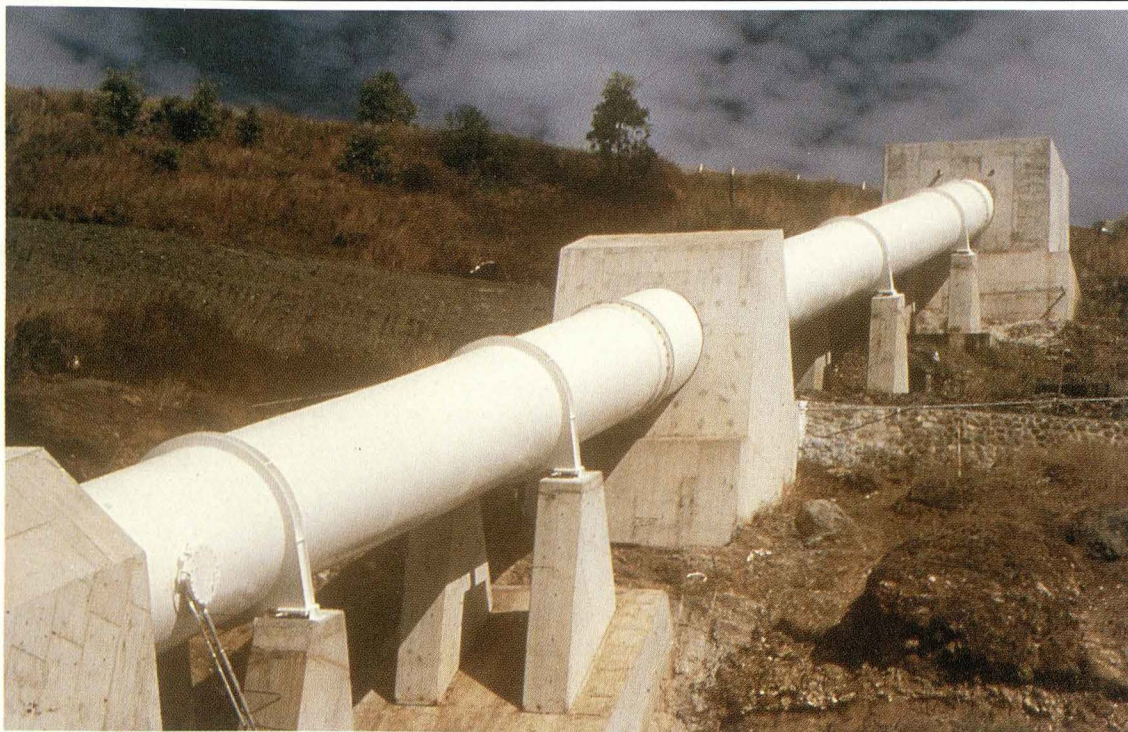
A section of Rouna 4 Penstock, near Port Moresby. 2.2 metres diameter, 300 metres long. Internal surfaces treated with 400 micron film thickness of Tarsel, Standard tar epoxy. External surfaces 75 micron film thickness of Dimetcote 5, inorganic zinc silicate and 75 micron of Unilite 400, poly vinyl chloride. Application by: Hornibrook Constructions Pty Ltd.
