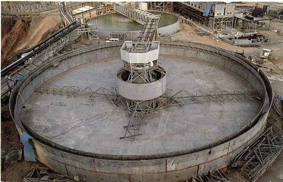
One of two 50 metre diameter filtration tanks under construction for OK Tedi Mining Limited. Internal and external surfaces of the tank and structural steel treated with 75 micron of Dimetecote 5 inorganic zinc silicate primer after abrasive blast cleaning of the surfaces to class 2½ in accordance with AS 1627-4. Application by Hornibrook Construction Pty.Ltd.
