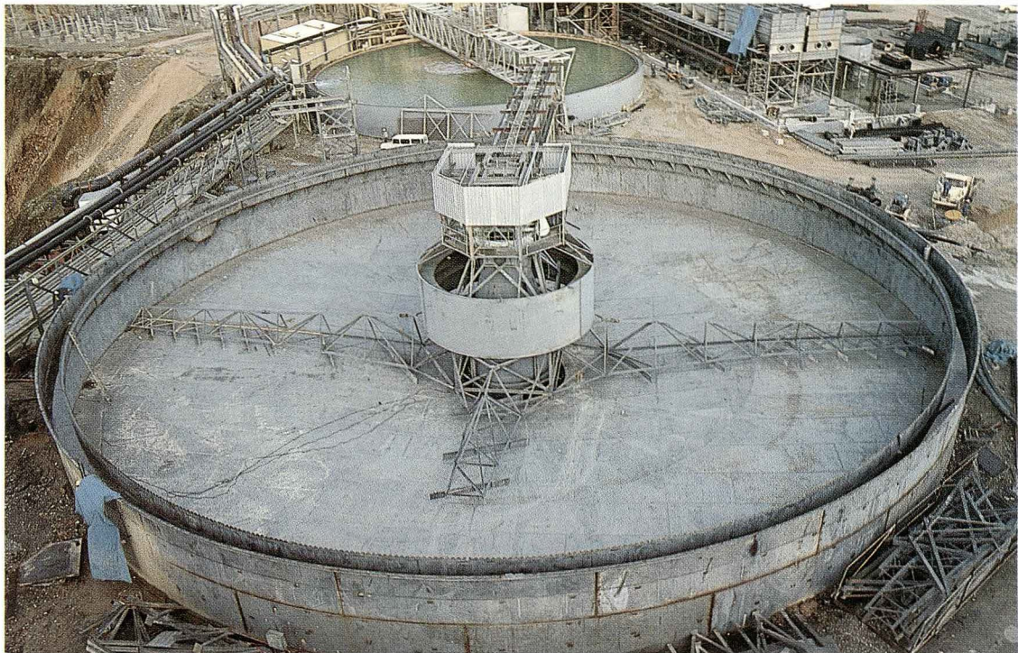
One of two 50 metre diameter filtration tanks under construction for OK Tedi Mining Limited. Internal and external surfaces of the tank and structural steel treated with 75 micron of Dimetcote 5 inorganic zinc silicate primer after abrasive blast cleaning of the surfaces to class 2½ in accordance with AS 1627-4. Application by Hornibrook Construction Pty.Ltd.
