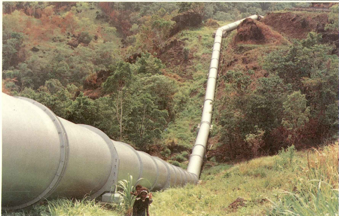
A section of the Rouna 3 water pipeline near Port Moresby. External surfaces treated with Amerlock 400 high build epoxy mastic applied in two coats to 250 micron dry film thickness.
