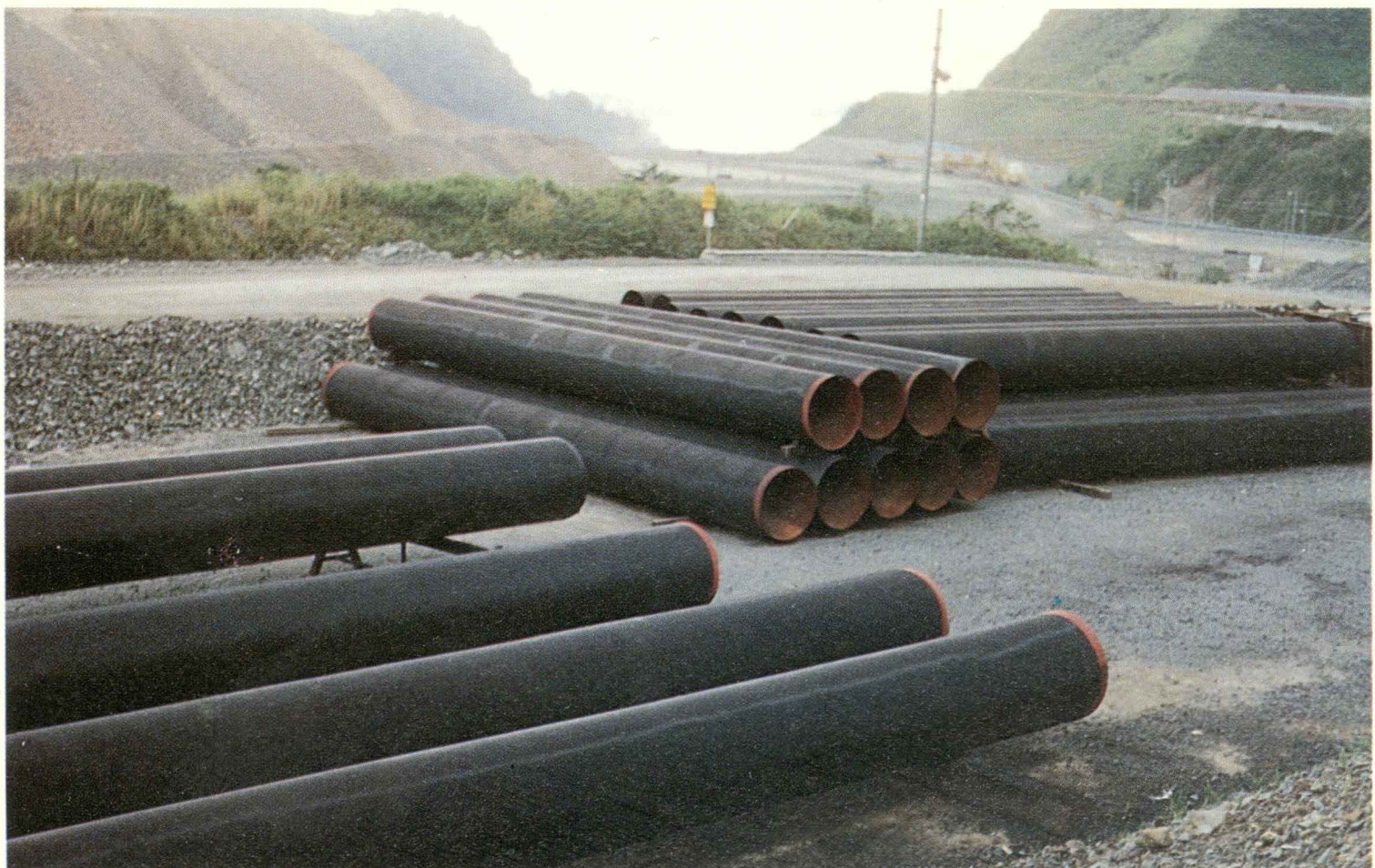
"A portion of a large quantity of steel water supply pipes for Bougainville Copper Ltd., Panguna, externally treated with Dimet Tarsset Standard High Performance Tar Epoxy, to 400 micron dry film thickness. Application by Minenco Pty. Ltd."
