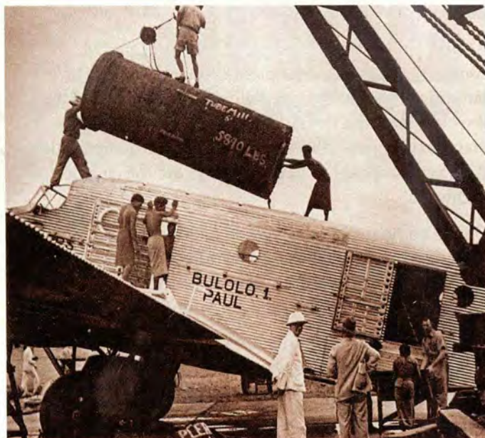
The Junkers G31... big enough for any dredge but a hatch had to be cut into the roof of the fuselage to handle some awkward pieces.
