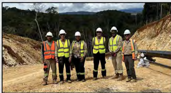
ExxonMobil PNG Chairman and Managing Director, Peter Larden (third from right), meets with the Angore Project Pipeline and Construction team.
