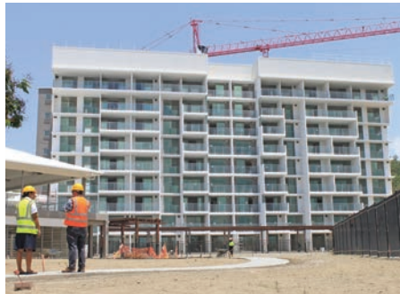
Ground breaking ... Air Niugini's residential building will include a restaurant and gym open to the public.
