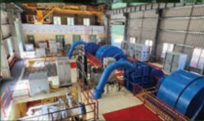
Sneath Hydro Power Station, Balme
